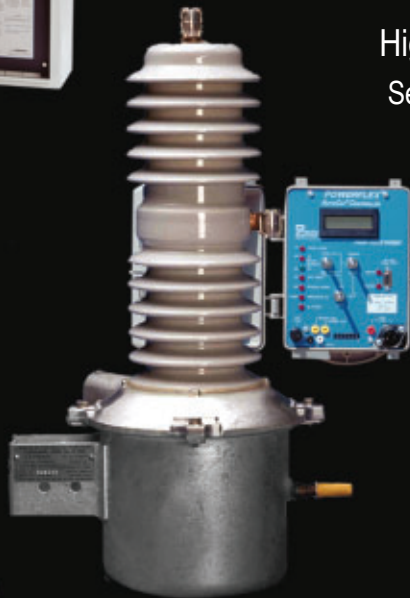
Voltage/Var Management Capacitor Switches & Controls
